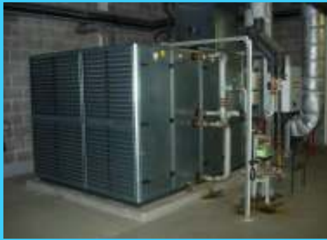
◀ Air handling unit installed at Swansea Bay.
